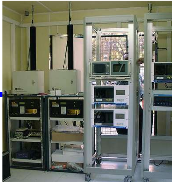
Monitoring Station (Interior View)
